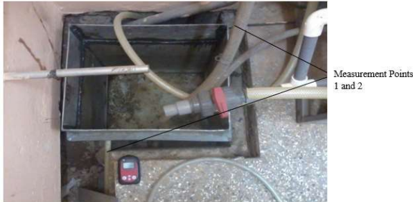
Fig. 4. Deionizer room showing measurement points 1 and 2 of the inlet tank that connects to the irradiation chamber through the concrete walls
