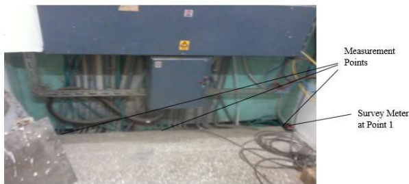
Fig. 3. Electric room showing measurement points
