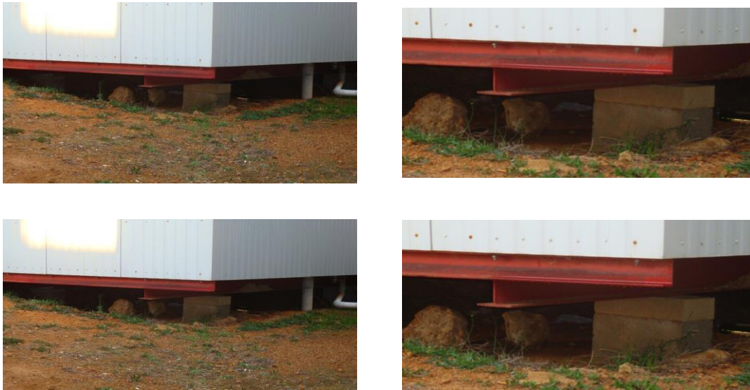
FIGURE 5 Plate 6 and 7. Buildings Undermined by Rainwater-Induced Soil Erosion
